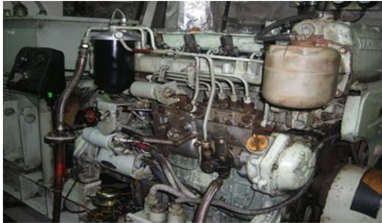
Figure 2. Main engine (Example of field survey documentation)
